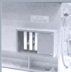
Auxiliary Box with cover removed but the different voltages separated by "Box within a Box" on the right side.
