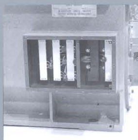
"Box within a Box" with cover removed.
